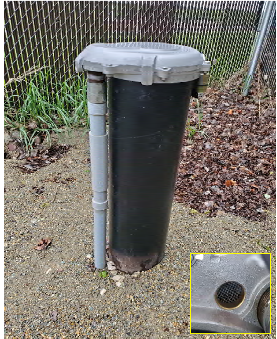
Well-2 (WL003): Well-2 is the new well which was installed in 2020. It is positioned off the NE corner of the Pump house. It also employs a turtle style wellhead cap which was secure, sealed, and properly vented (picture insert). The conduit servicing the well was also secure and free of defects.
