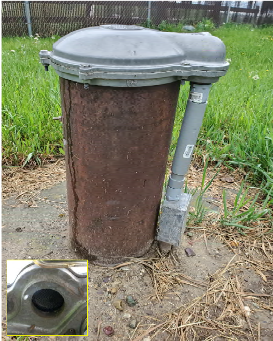
Well-1 (WL002): Well-1 is positioned between the pump house and the storage tank. It employs a turtle style wellhead cap which was secure, sealed, and properly vented (picture insert). The conduit servicing the well was also secure and free of defects.
